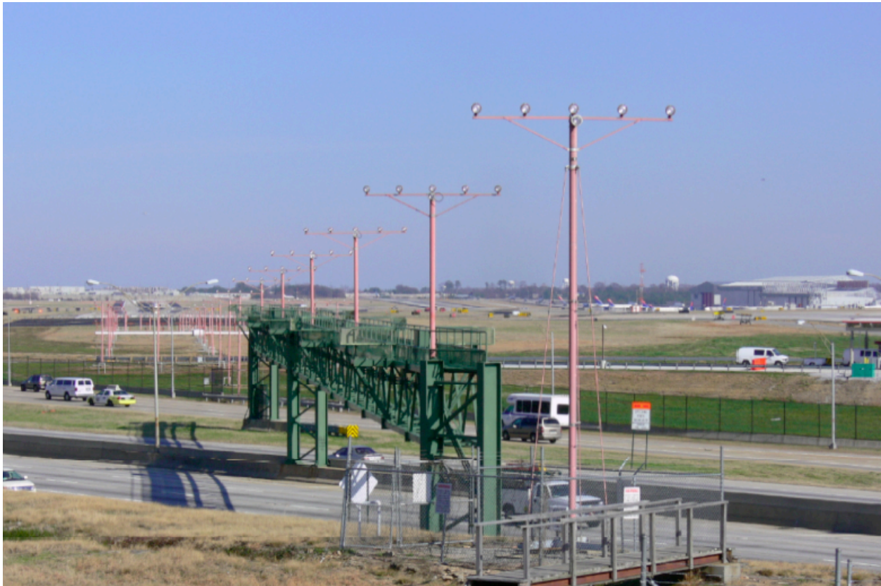
Figure 1. ALSF2 Runway Approach Light System Deployed at Atlanta Hartsfield International Airport.
